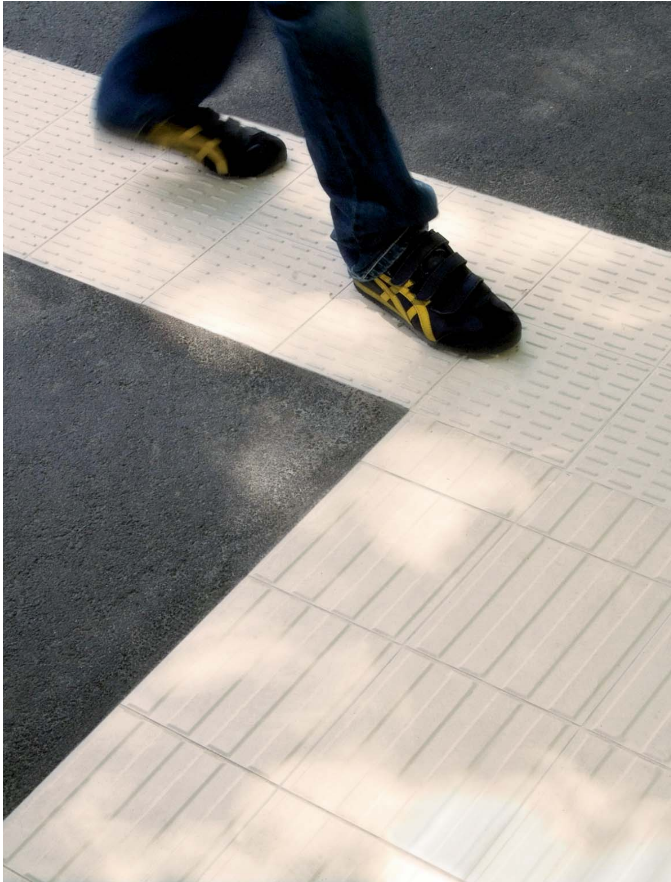
Bus Stop, Merano, Italy. Project: Studio A4 KXWU Attention Service Code 20x20 KXWS Straight Direction Code 20x20
